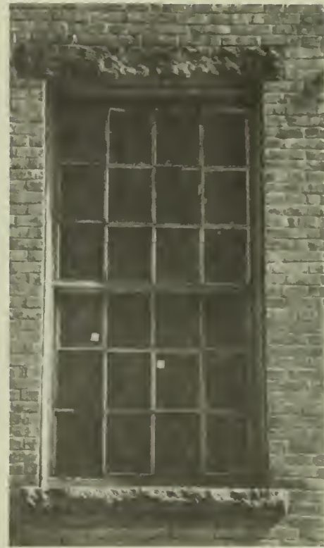
Figure 2. Because of the historic character and significance of the complex, replacement sash needed to have true divided lights and the dimensions and profiles of visible elements needed to be close copies of the originals. Photo: Courtesy of Huygens DiMella Shaffer
